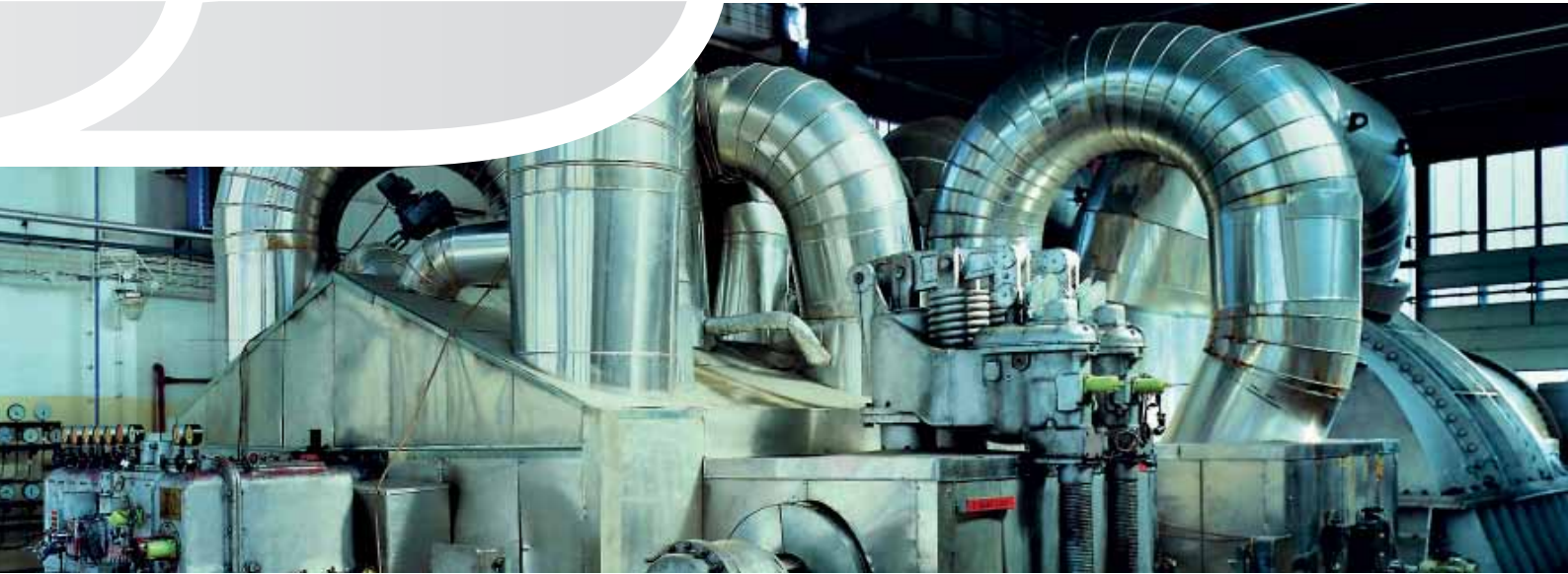
CEZ GROUP - Coal-fired power plant in Počerady, Czech Republic
