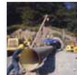
pg. 109 Laying of the oil pipeline, Val Aupa (Udine) Photograph (1973) courtesy of ENI Historical Archive, Rome
