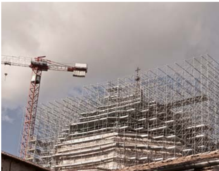
Above and on page 5: Reconstruction in L'Aquila, destroyed by a violent earthquake on 6 April 2009 (a series of seismic events began in December 2008 with epicentres all over the city, the L'Aquila Basin and parts of the province, as well as other areas of Central Italy)
